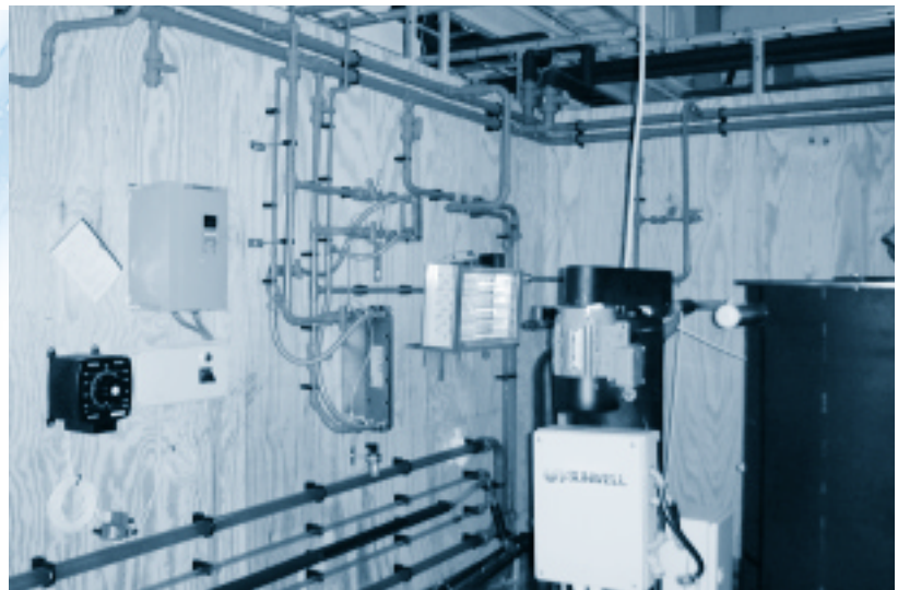
Test facility for component trials and for the determination of heat transfer coefficients.
